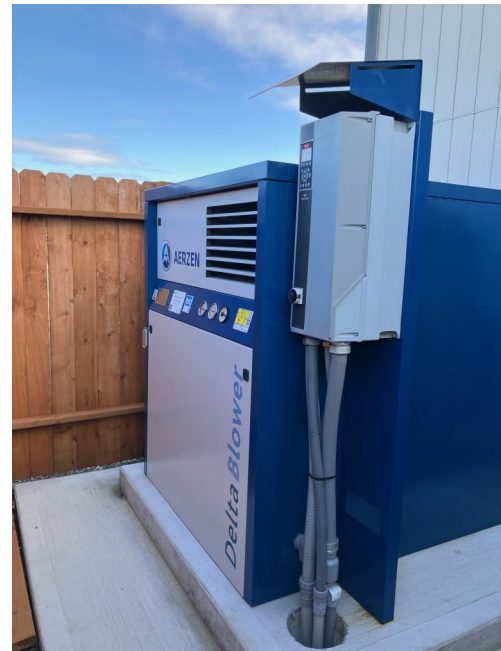
Photo: Treatment plant blower
